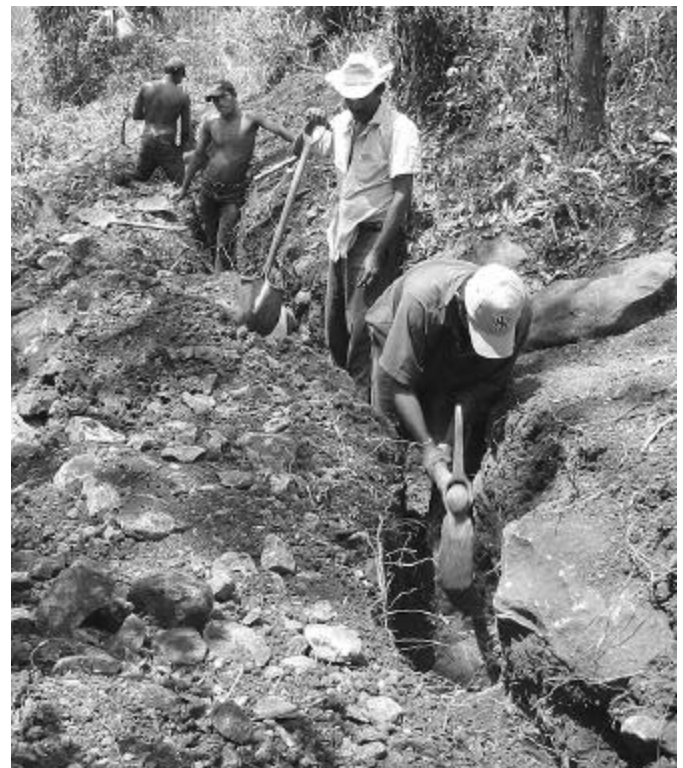
Villa Siquia community members dig the trench for their water system through very rocky soil.
